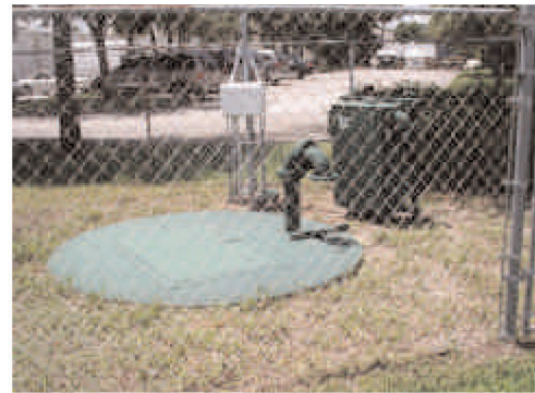
Lift Station Odor and Airborne Bacteria control
